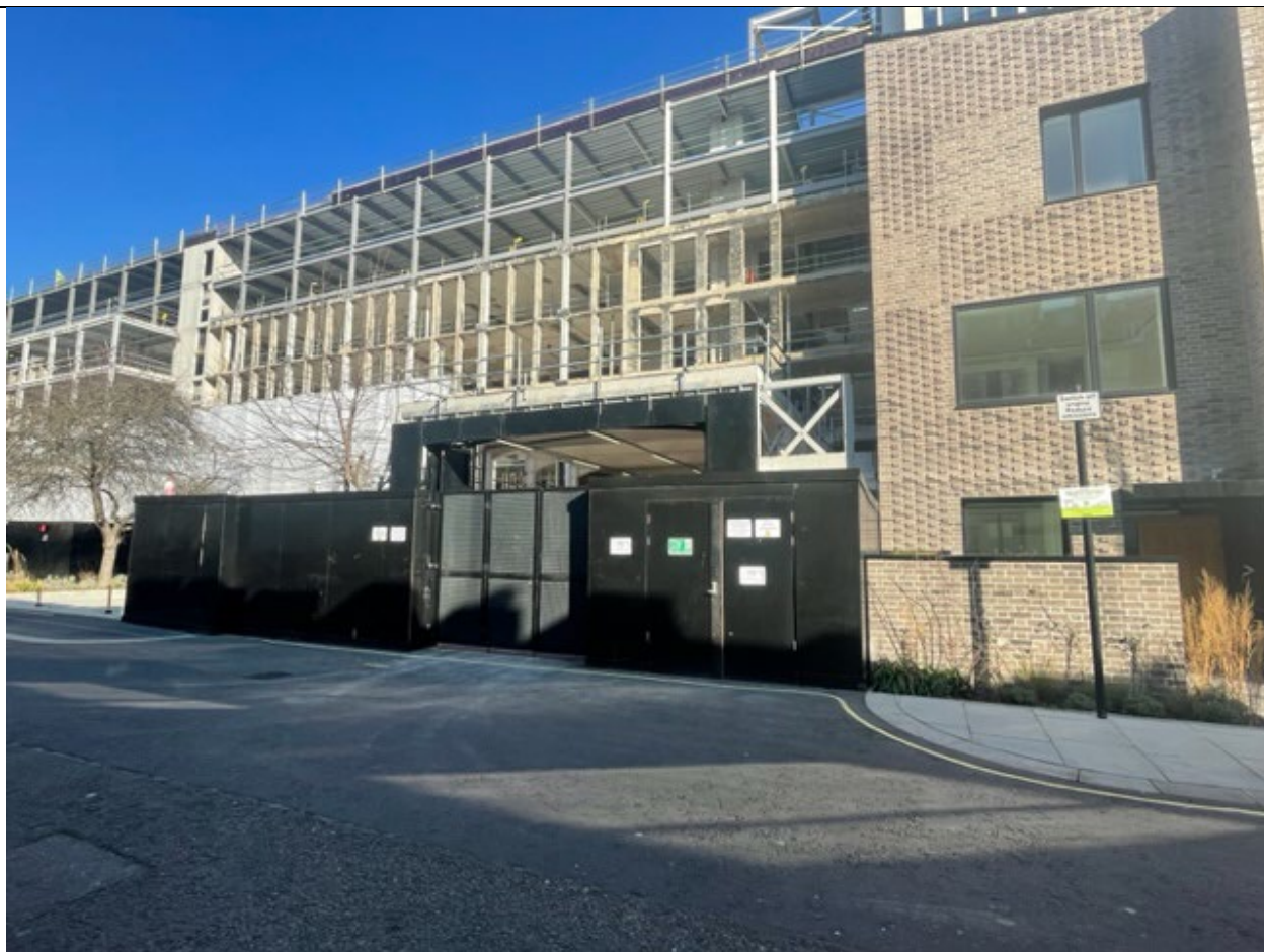
Loading Bay for 50 Eastbourne Terrace (& 40 Eastbourne Terrace) under construction in Chilworth Mews.
